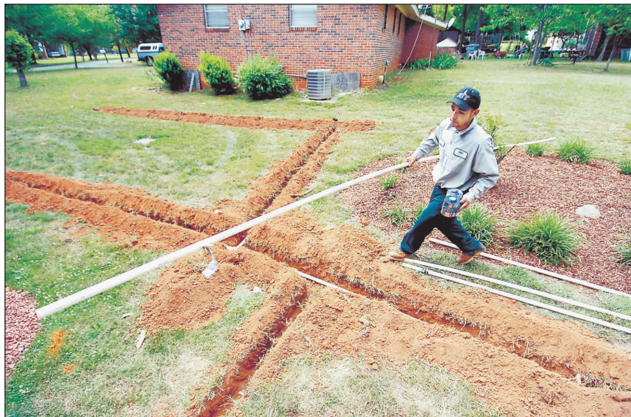
Juan Rodriguez of AllGreen Irrigation and Landscape installs pipe at a residential site in Charlotte on Wednesday afternoon. The use of sprinkler systems in commercial and residential development is growing in the area.
